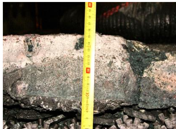
Figure 5. Cross-section of a smelt bed in a boiler with floor tubes covered with lime in the previous outage
