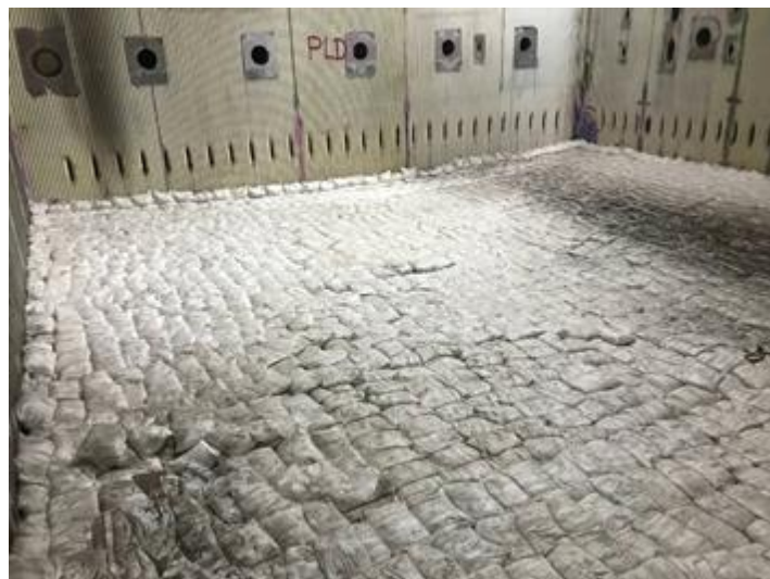
Figure 1. Recovery boiler floor covered with sodium sulphate bags
