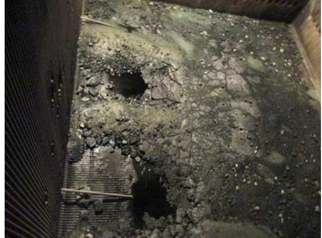
Figure 6. Floor after smelt extraction and washing in a 2500 tDS/day recovery boiler
