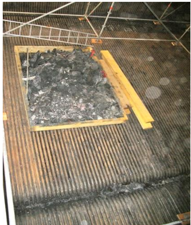
Figure 7. Cleaned floor in 2017 outage after smelt extraction and enhanced floor washing when no material was used for floor protection
