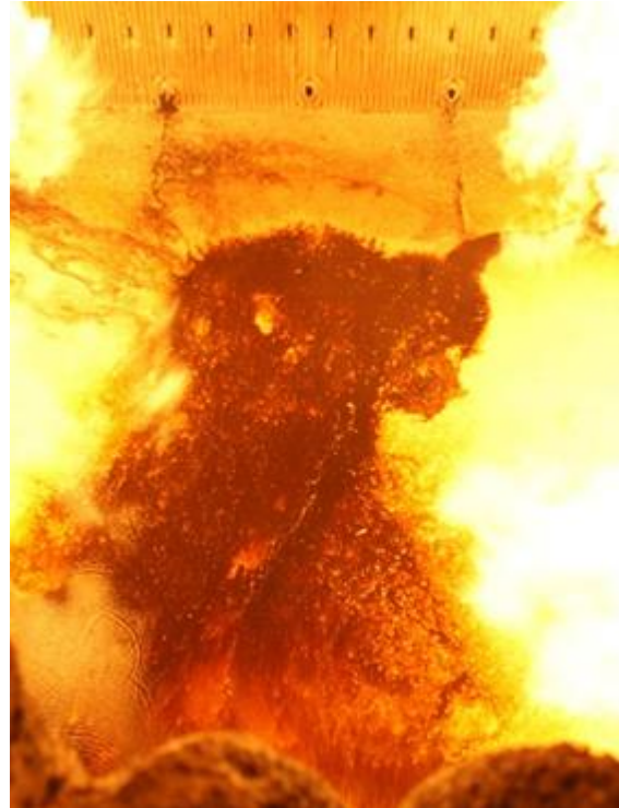
Bed remaining on the floor after smelt extraction, when lime had been used as floor protection material in the previous outage
