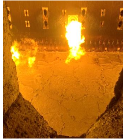
Figure 2. Recovery boiler floor covered with sodium sulphate solution (after dry-out)
